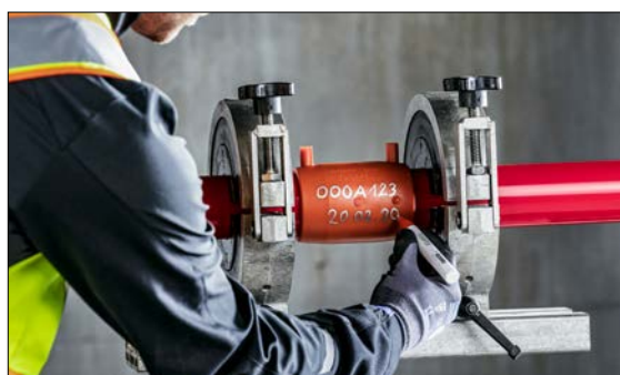
Fig. 03-18 Record the personal identification number and the current date on the electrofusion fitting with a marker pen.
