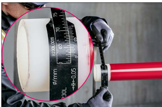
Fig. 03-6 The diameter must not fall below the permitted minimum diameter (as per Tab. 03-3). Before carrying out any further required scraping, check whether the current outer diameter would allow an additional scraping (swarf thickness: 0.1 to 0.3 mm, depending on the rotary scraper). If necessary, remove residual colour with a hand scraper.
