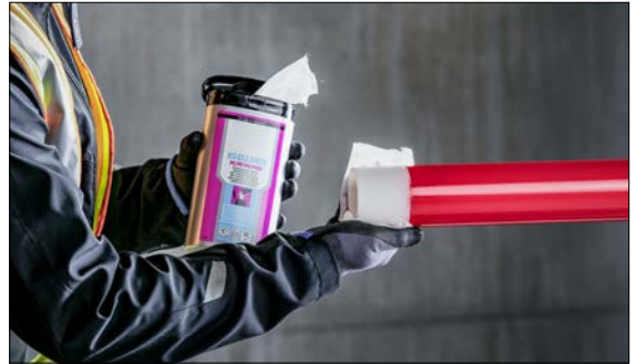
Fig. 03-8 The scraped section must be free of dust and grease. Clean with sufficient Tangit cleaner and let it evaporate completely.
