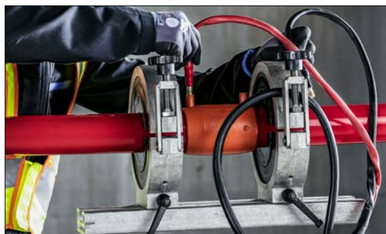
Fig. 03-16 An audible double signal can be heard if the welding process was successful. "OK" is shown in the display. The plugs can be removed.
