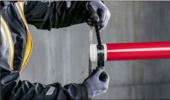
Fig. 03-7 Check the pipe end prepared for connection using the circumferential measuring tape if necessary.
