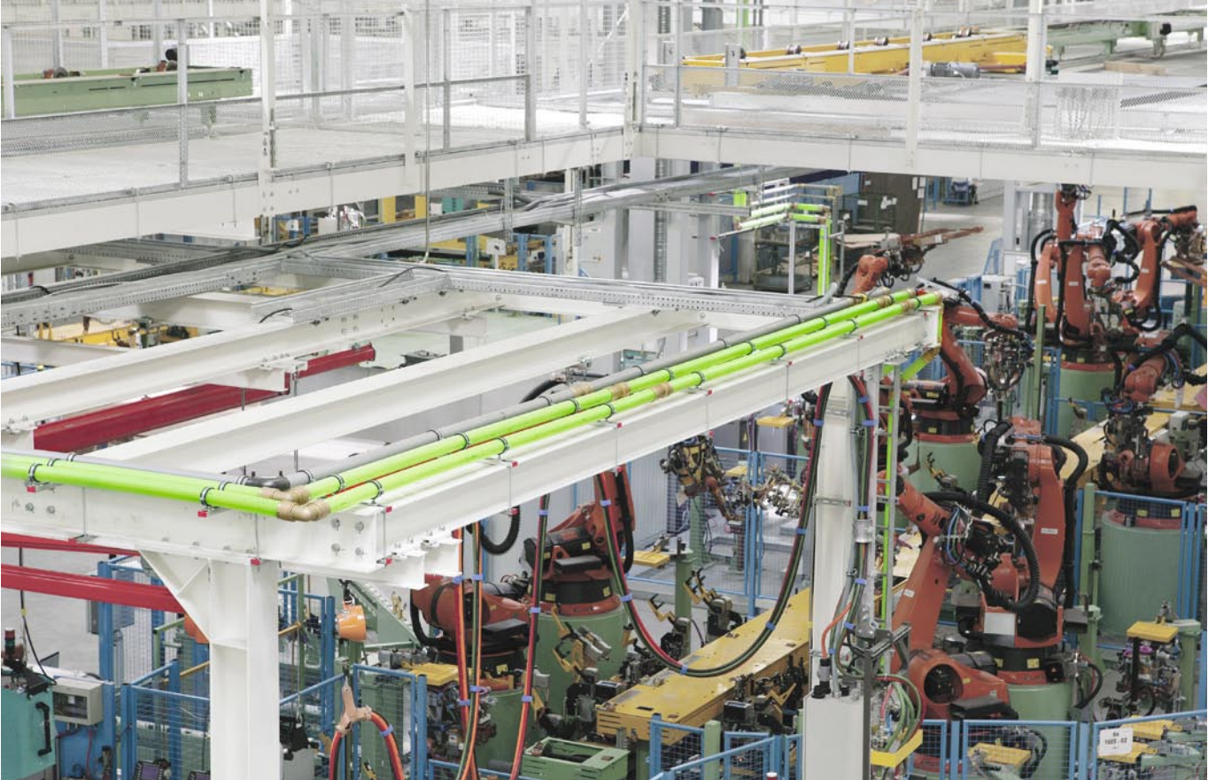
DaimlerChrysler AG: Providing welding robots with compressed air and cooling water.
