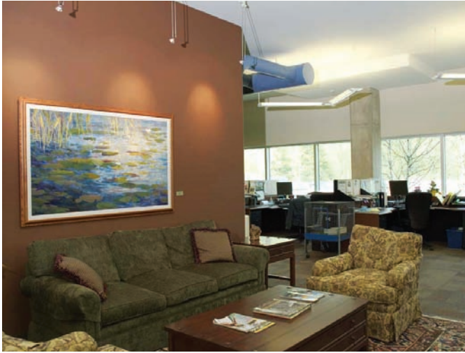
Specifiers integrated the engineering functionality of an exposed concrete radiant-cooled ceiling with the architectural vision of exposed ductwork and drop lighting to provide a collaborative feel within the interior space at Earth Rangers Centre (ERC) in Woodbridge, Ontario.
