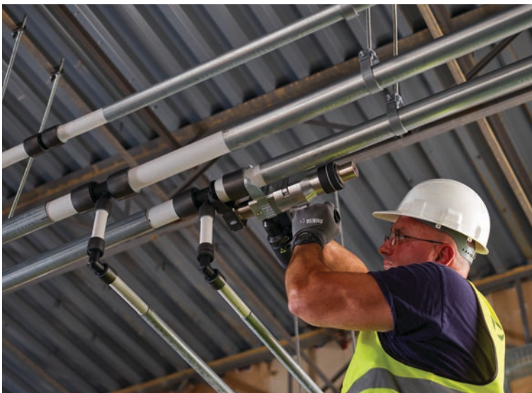
Plumber using PEX expansion/compression tool to form secure connections in commercial project. Also shown are galvanized steel support channels and support hangers.
