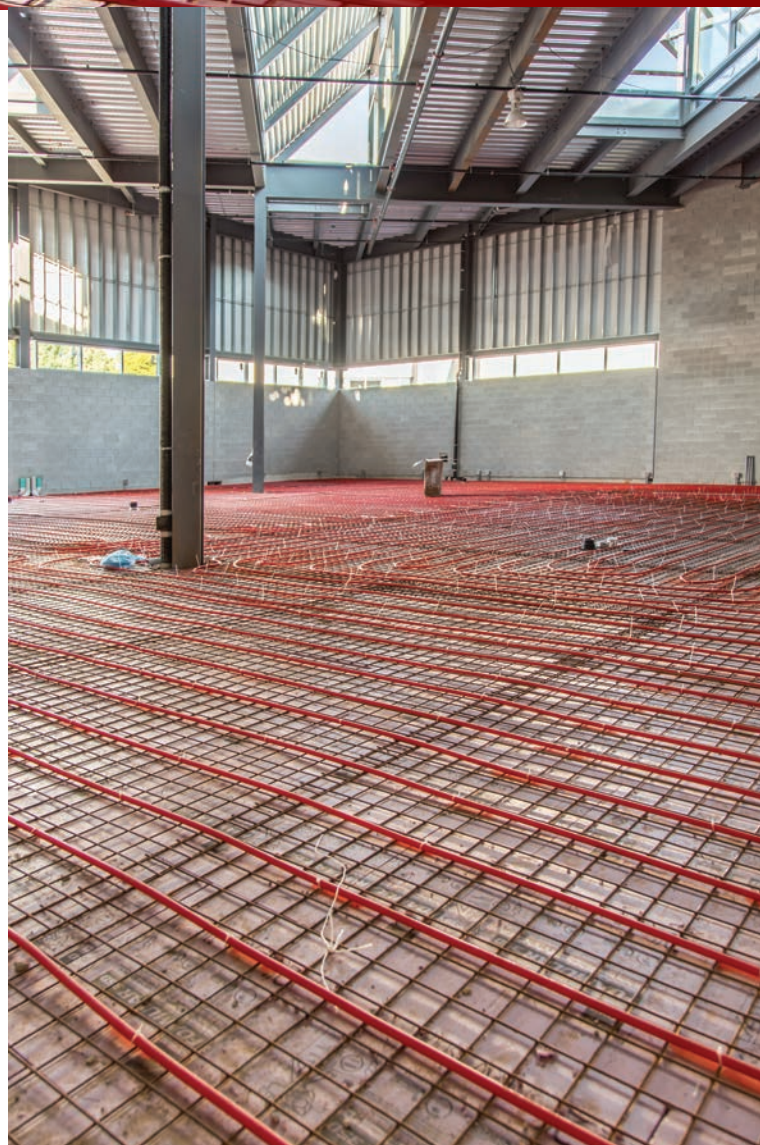
Radiant heating/cooling system being installed in Sheridan College Skilled Trade Center. (source: Klimatrol Environmental Systems Ltd.)
