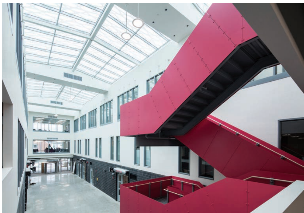
Radiant heating/cooling has been combined with DOAS at Sheridan College Davis Campus (Brampton, Ont.). Pictured: the three-story atrium at the Skilled Trade Centre. (source: REHAU)
