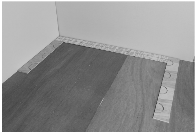
Fig. 6: Lay out header row and return bends for floor installation, ensuring square
