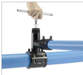
Fig. 61 9. At the conclusion of the pressure test, use an NW 12 Allen key to screw the hollow punch into the main pipe.
