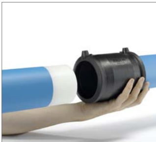
Fig. 46 8. Prepare the second pipe end, then slide it completely into the electrofusion fitting.
