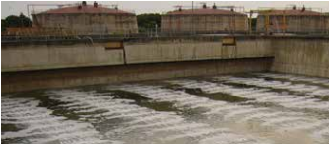
Shah Alam STP (Malaysia)
