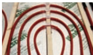
IMPORTANT Pipe bends are laid in light bulb shape
