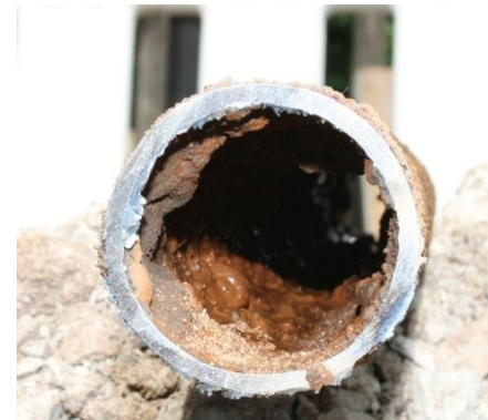
Unpleasant discovery: A removed metal pipe section with incrustations.
